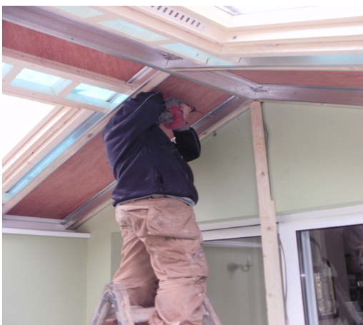
6. Gable rafters to be secured to the house wall using suitable fixings depending on wall
