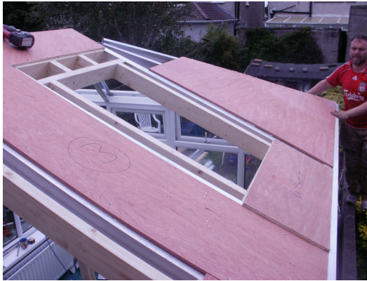
7. Fix timber sheets to rafters using self tapping screws at 200mm centres
