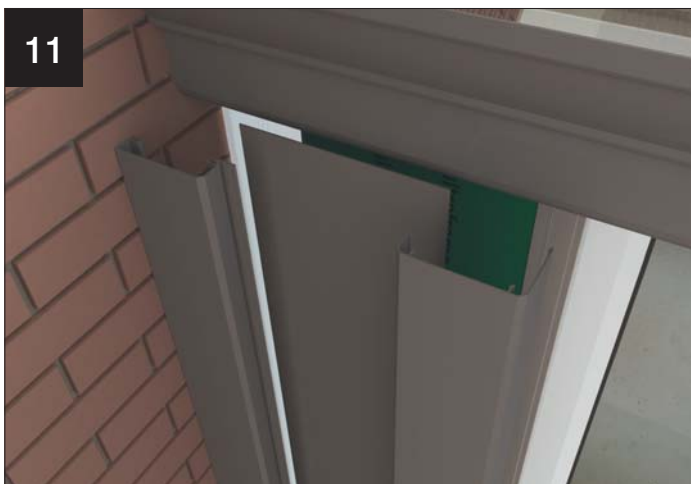
Now complete the cladding sequence on the abutment column – attaching cleats, then the full height cladding and infill panel ( similar to step 3).
